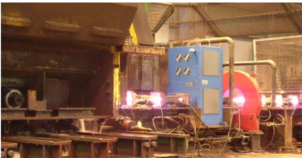
This commercial system is installed in a bar mill that rolls steel bars ranging in diameter from 0.5 in. to over 1.5 in. The HotEye™ system is the blue unit visible towards the right in the picture.
